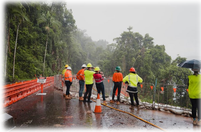
Regional Road & Transport Group Technical Committee Technical Tour September 2025 – TMR Landslip at Daintree Village
