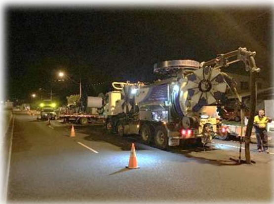
Figure 13 Works on sewers at night are sometimes required for high-flow sewer to minimise disruption to residents.
