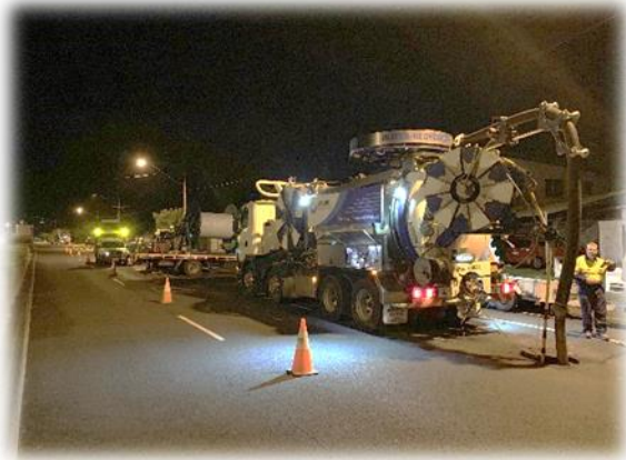
Works on sewers at night are sometimes required for high-flow sewers to minimise disruption to residents.
